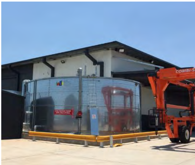
Source: Northline Plate 3-13 Example of rainwater tank
