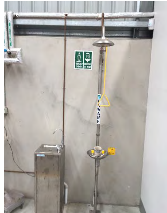
Source: GibbGroup Plate 3-11 Example of emergency shower and eye wash station
