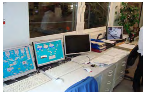
Plate 3-8 Control room of typical hydraulic backfill plant
