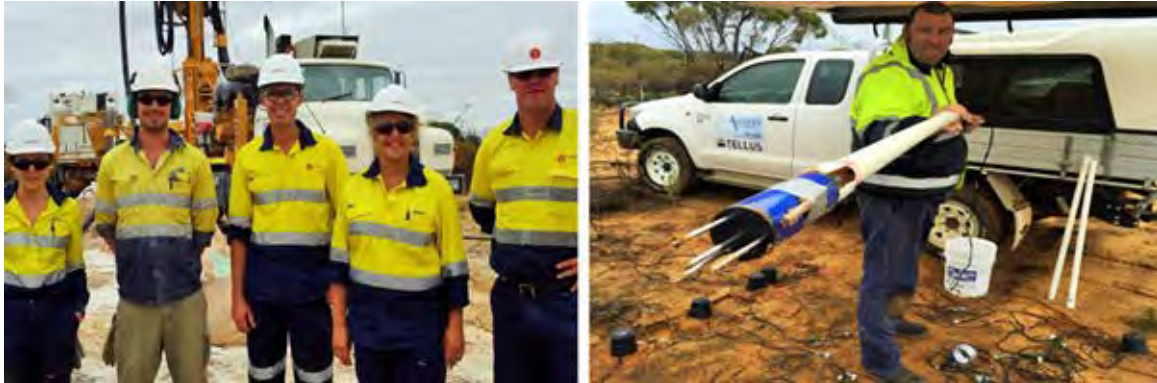
Seven monitoring bores were drilled to confirm the absence of groundwater (left). Equipment was installed to confirm soil evaporation rates (right).
