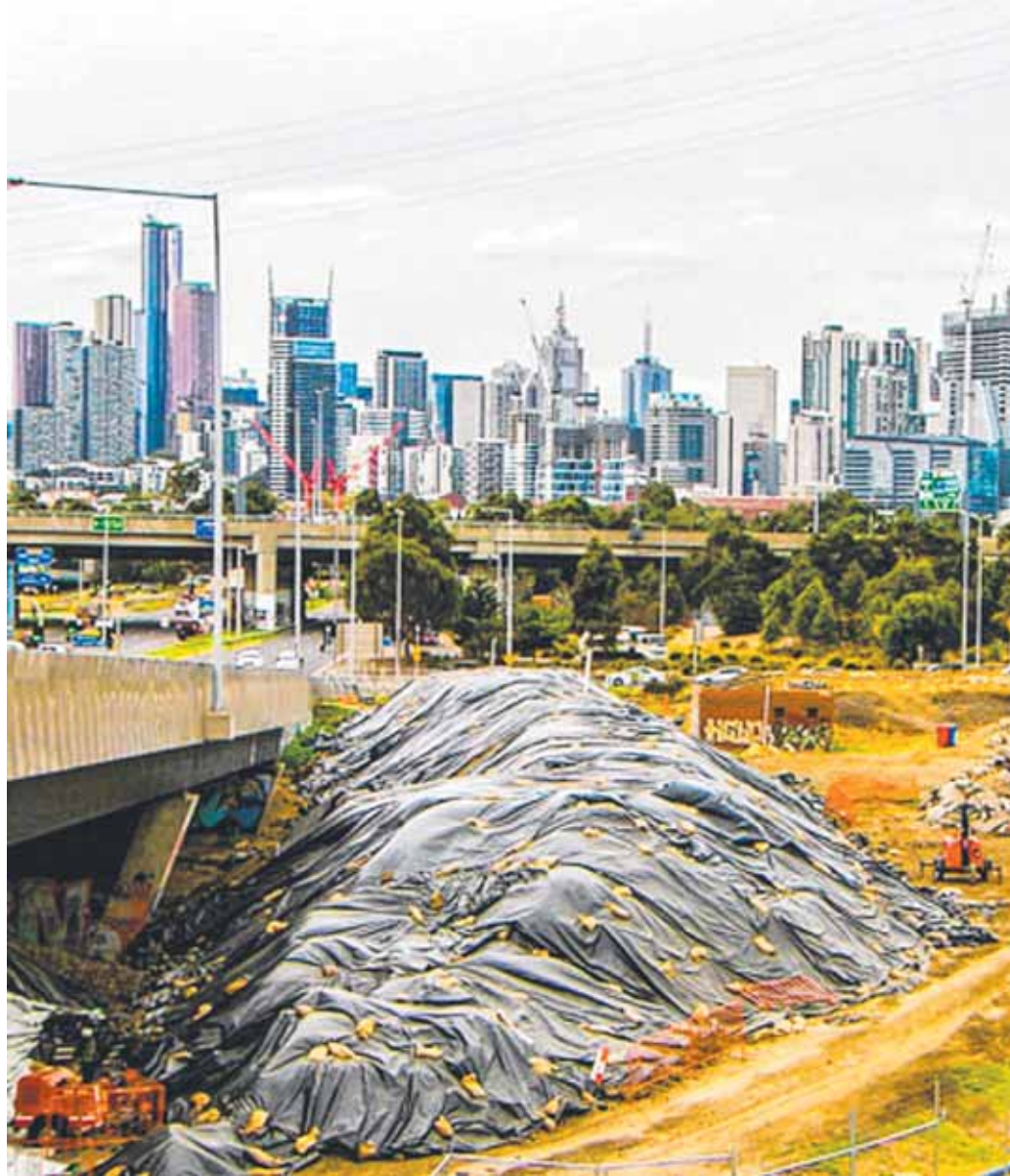
Asbestos, chemicals and other toxic waste on site at the West Gate Tunnel project
